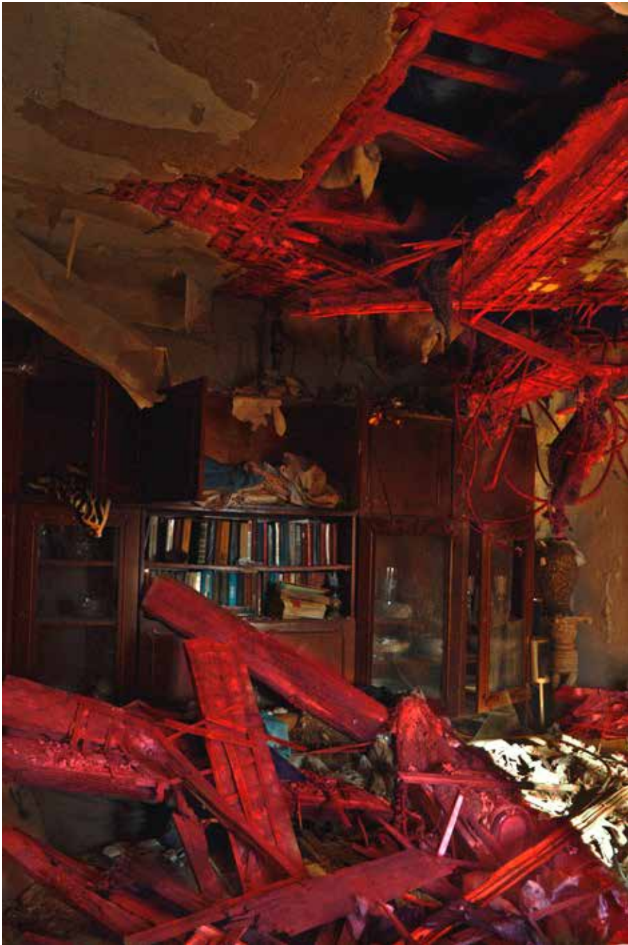
The destroyed room of my house. A fragment of a rocket under the rubble. Cherkasy Tyshky
